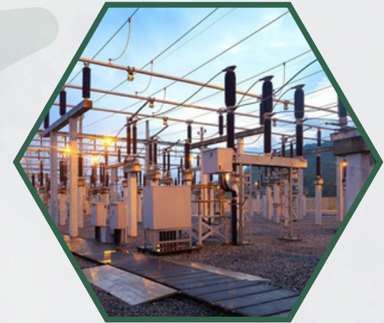
Utilities and Basic Infrastructure Services
